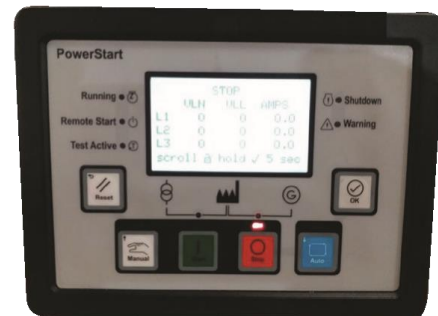
PowerStart 600 control operator /display panel
